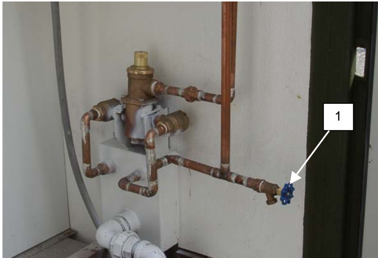
Containerized Shower with Copper Plumbing
